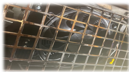
Delray E-Fan mounted behind 57" T-Bird
